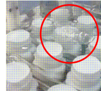
Visual leak detection
